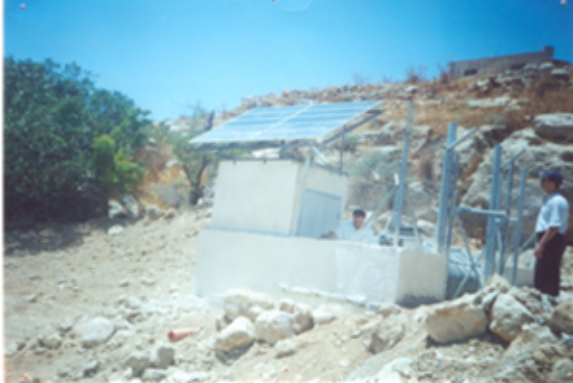
Figure 7: PV water pumping system, Yanoon village
