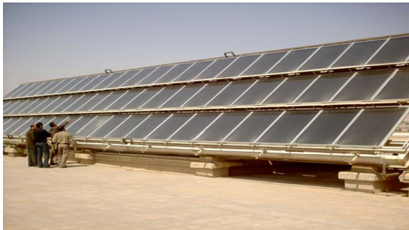
Figure 6: Collective Solar system at Jericho hospital
