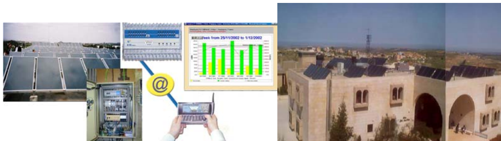
Figure 5: Collective Solar system at Beir Zeit University
