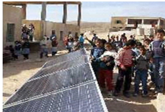
Figure 10: School PV system
