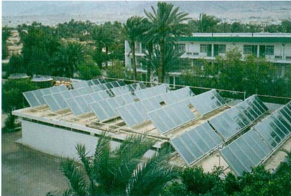
Figure 57. Solar collectors of the Coral Beach Hotel in Aqaba [source: NERC]
