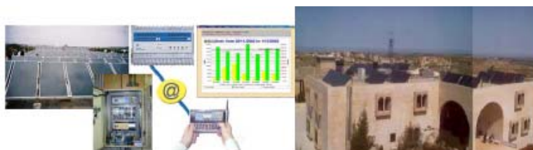
Figure 54. Central solar thermal system in Beir Zeit University, in the Palestinian Authority [source: PEC]
