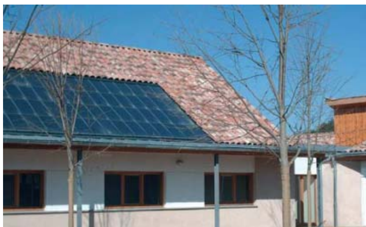
Figure 41. Solar panels integrated on the roof of the Oraison public retirement home [source: ADEME]
