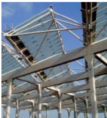
Figure 43. Roof of the Besós sewage treatment plant with 600kW photovoltaics in Barcelona [source: IDAE]
