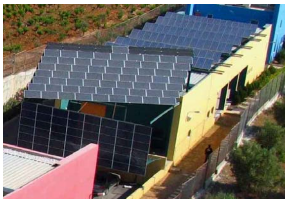
Figure 53. The 22kWp PV installation on the roof and wall of the laboratory of PV technology in CRES [source: CRES]
