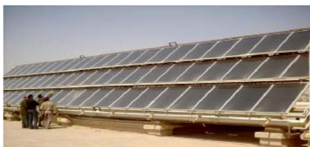
Figure 55. Central solar thermal system in Jericho hospital, in the Palestinian Authority [source: PEC]
