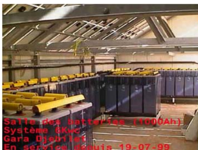
Figure 47. Batteries of PV systems in Gara Djebilet [source: APRUE]
