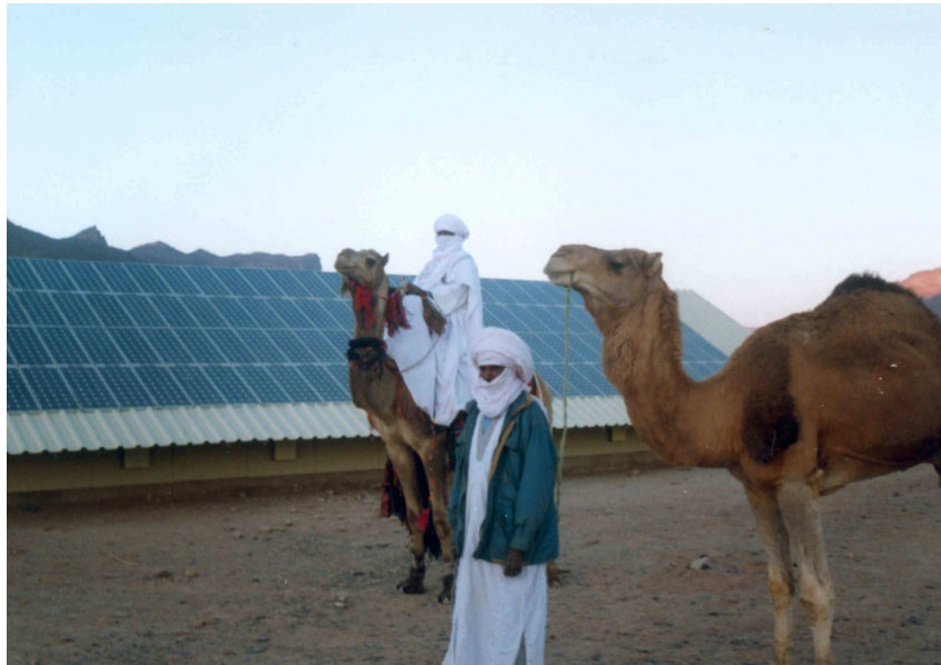
Photovoltaic panels The electrification of 20 villages in the great Algerian south
