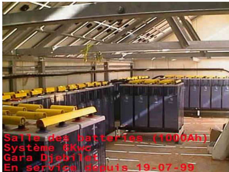
The batteries room, in function since 1999 The electrification of 20 villages in the great Algerian south
