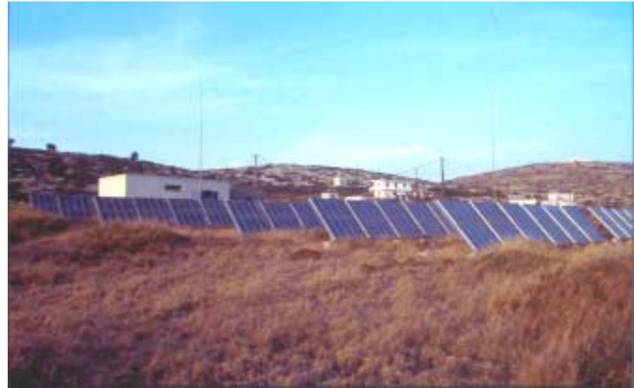
27.5kWp PV System at Arki island
