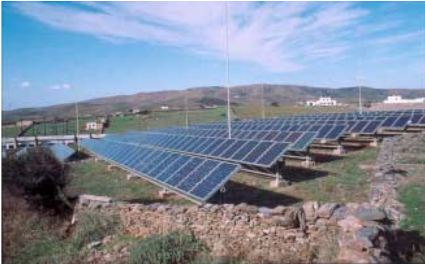
100kWp PV System at Kythnos island
